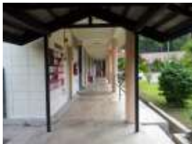
a) Corridor (but no drain cover)
