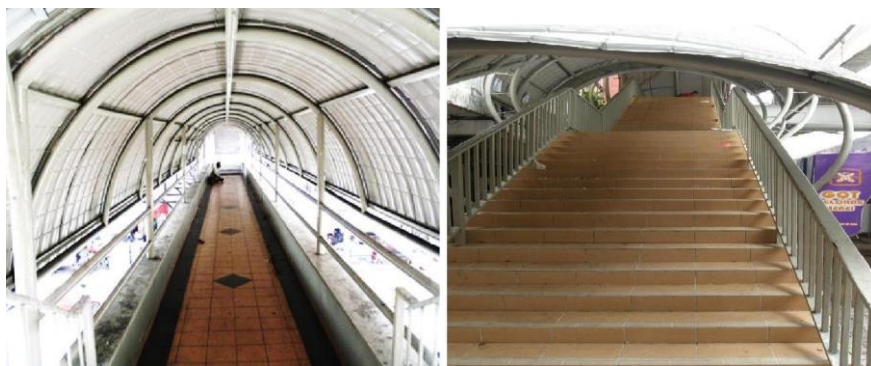
Figure 4: Overhead crossing in Jalan Tuanku Abdul Rahman that is isolated from the pedestrian route (Source: Authors)
